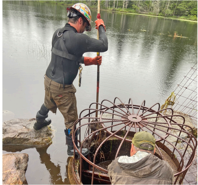
Crew working to remove accumulated beaver debris from "moose bog" pond outlet control structure to ensure waterflow downstream.
