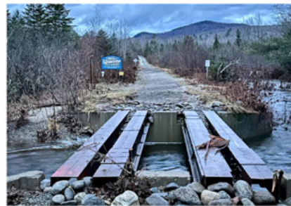
Top row: Huston Brook Bridge storm damage left is May 1st, Right is December 18th. (photo’s courtesy of Tom Cromwell)
