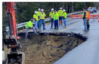
Bottom row: Redington Bridge views from the December 18th, 2023, storm damage.
